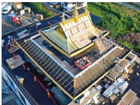
The bird's-eye view of Thrangu Monastery Canada under construction 加拿大創古寺在建設中之鳥瞰圖
